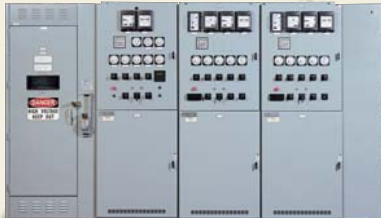
This Switchgear is also shown on the cover.
